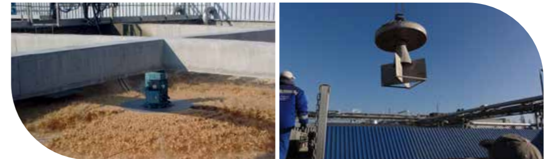
industrial wastewater treatment / pharmaceuticals / SBR / two-stage system / 280 m 3 treated wastewater on a daily basis
